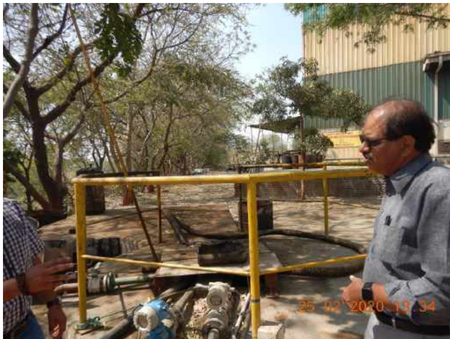
Plate 7.5.4: Effluent treatment facility at GEPIL, Alang
