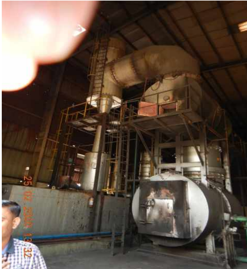
Plate 7.5.3: A view showing incinerator installed in GEPIL at Alang
