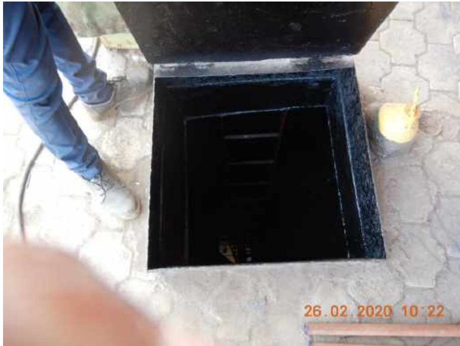
Plate 7.3.5: A photo showing collection pit constructed to collect oily waste
